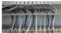
CABLE FIXING CROSS MEMBERS
